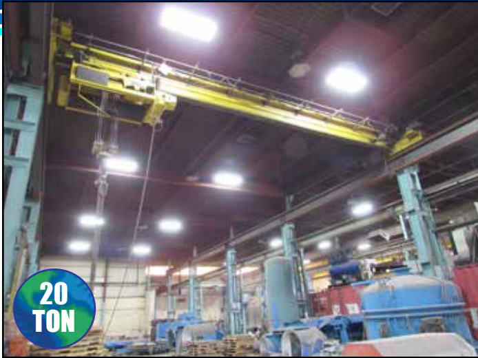
NORTH AMERICAN 20 TON OVERHEAD CRANE
