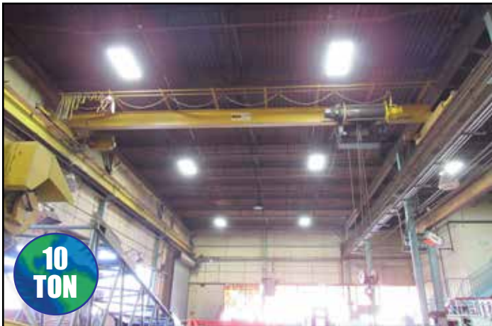
P&H 10 TON TOP RUNNING BRIDGE CRANE
