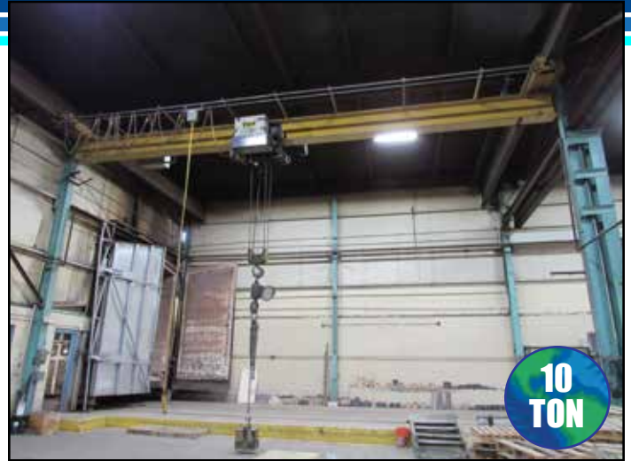
P&H 10 TON UNDERSLUNG BRIDGE CRANE
