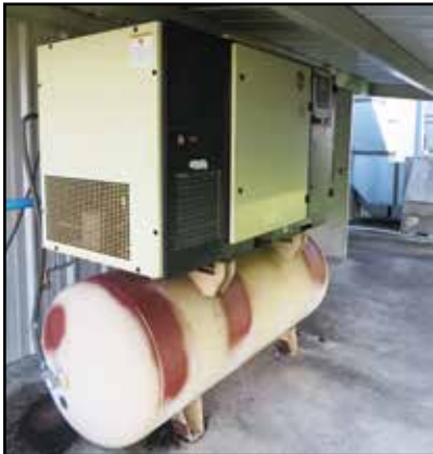
INGERSOLL RAND 20 HP TANK MOUNTED ROTARY SCREW AIR COMPRESSOR
