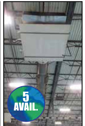
(5) PLANT AIR CONDITIONERS
