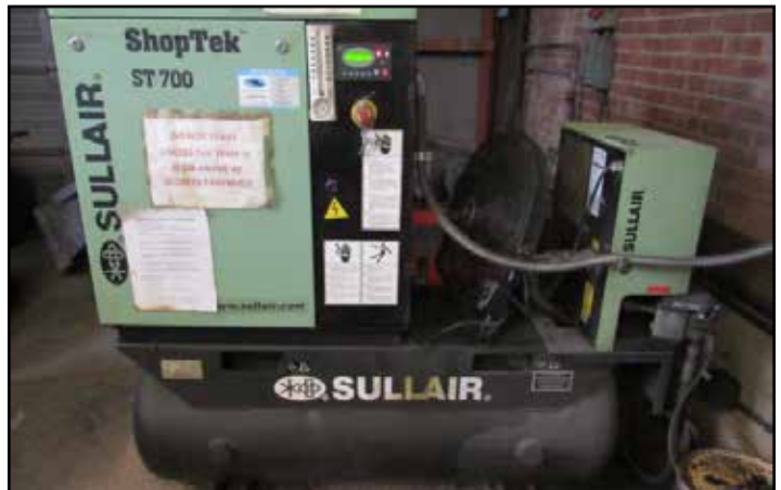
SULLAIR 10HP ROTARY SCREW AIR COMPRESSOR
