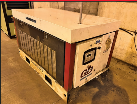
(2) 30 HP Gardner Denver Base Mounted Air Compressor
