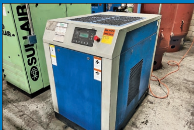
40 HP Kore Air Compressor
