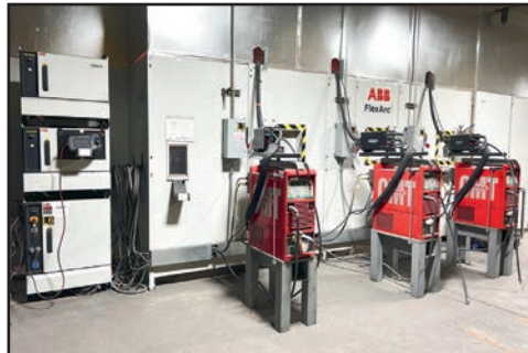
ABB WELD CELL-REAR VIEW
