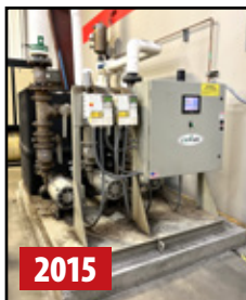
CONAIR PTS450 PROCESS WATER SYSTEM
