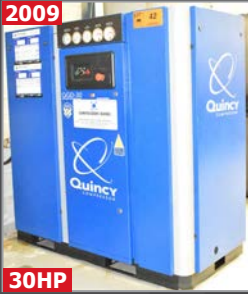
30HP QUINCY QGD-30-390528 rotary screw air compressor
