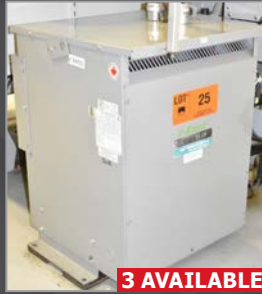
3 AVAILABLE Partial view of transformers available
