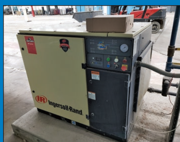
(10) Air Compressors 2HP to 50HP
