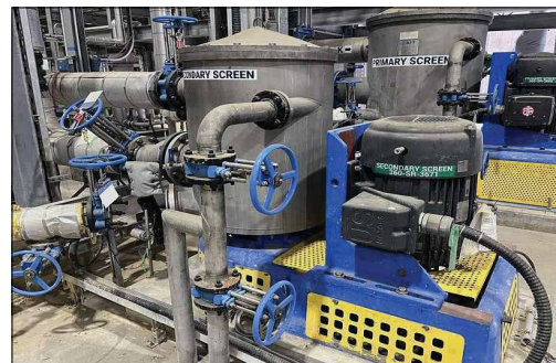
Bird M800 and M400 Pressure Screens Rebuilt by AFT in 2018
