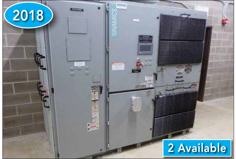
Siemens Perfect Harmony Drive 750 HP, Manufactured 2018, (2 Available)
