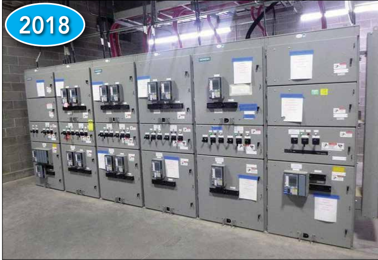
Switchgear SG-001 (with Arc Flash Detection) GM-SG, Manufactured 2018
