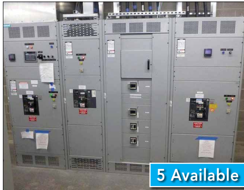
Siemens 480V Low Voltage Switchboard, Manufactured 2018, (5 Available)
