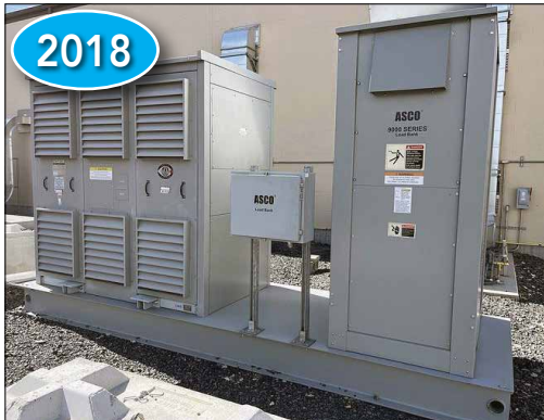
Asco 9000 Series Load Bank 1000KW, 480 Vac, 3PH 60HZ, with 1000KVA Mgm Transformer
