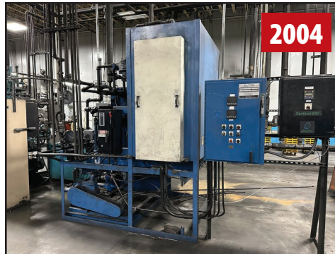
C. I. HAYES 3000 CFH EG RX GAS GENERATOR
