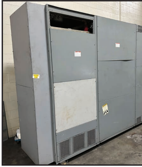
SQUARE D 3000 AMP SWITCHGEAR
