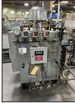
AJAX HIGH PRESSURE STEAM BOILER
