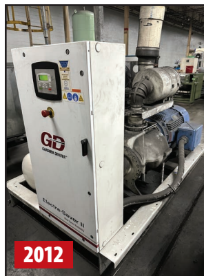
GARDNER DENVER ELECTRA-SAVER II 100 HP COMPRESSOR
