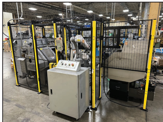
VIEW OF MACHINING CELL W/ ROBOT LOADING
