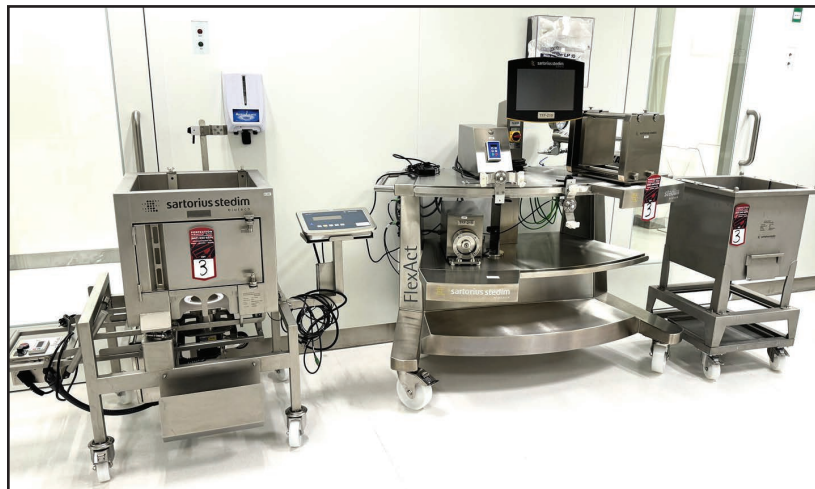
SARTORIUS STEDIM TANGENTIAL FLOW FILTRATION SKID
