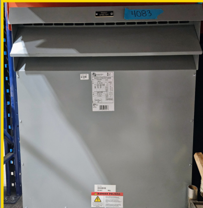
Multiple HAMMOND 112.5 kva Transformers
