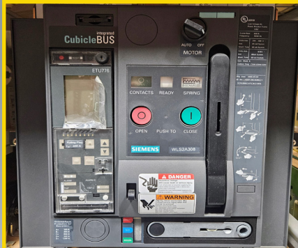
Multiple - CubicleBUS 800amp Breakers
