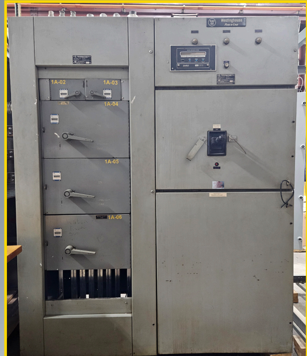
WESTINGHOUSE Pow-R-Line Switch Board 3000 amp w/ Fused Distribution
