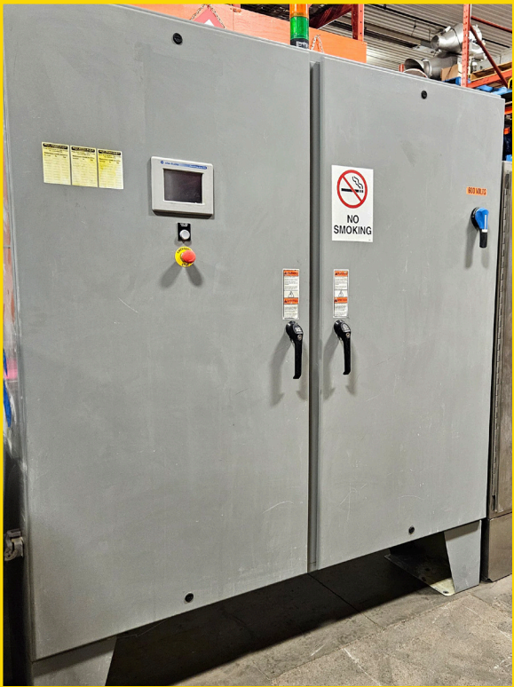
ALLEN BRADLEY Electrical Panel w/ Touch Screen
