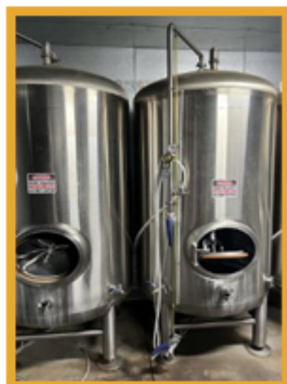
(8) Premier Stainless 15 bbl serving tanks
